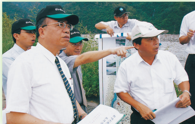
Control Yuan member inspect riverbank damage caused by July 2 inundation in Liukuei Village.
